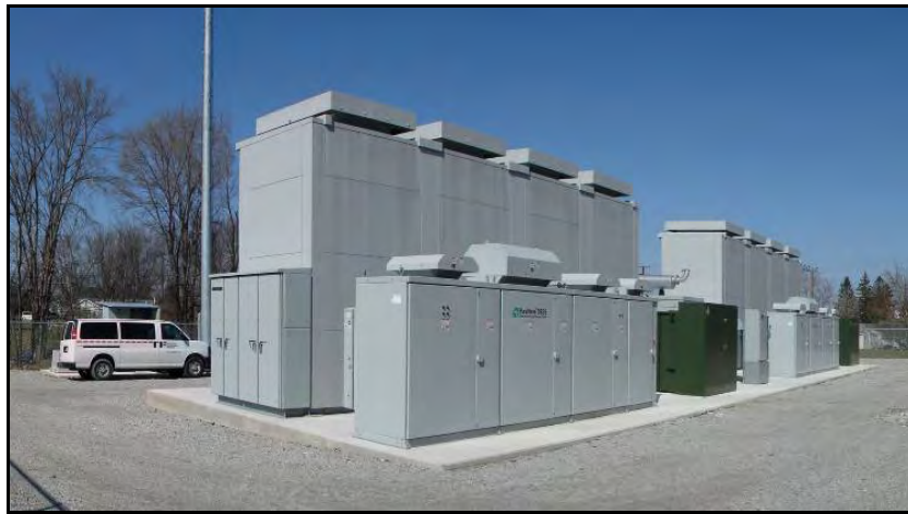
Figure 4-11 AEP Distribution Substation with Sodium-Sulfur Unit
